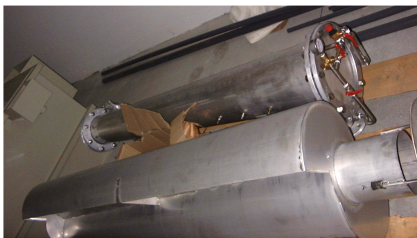
ULF detail sludge collection
