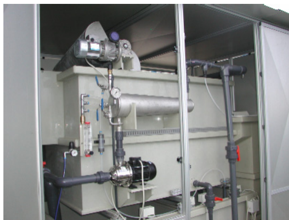
Spray box detail flotation machine
