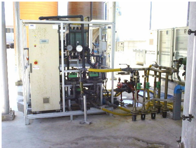
EDR overall view
