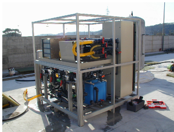
EDR installation phase
